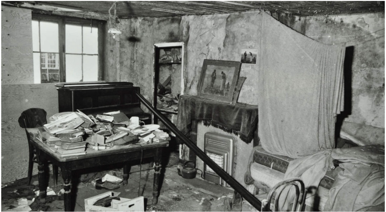
Interior of a house in Princelet Street : “View of bedroom of Grade II* listed terraced house at 19 Princelet Street, Spitalfields. Room in state of considerable disrepair, books, crockery, and furnishings are scattered throughout.”
