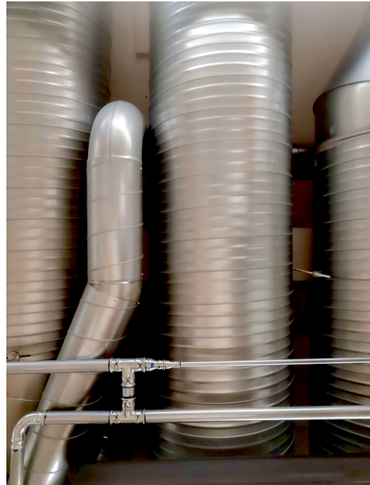
Fragment of ventilation system at KHiO. Photo credit: Dariusz Wojdyga
