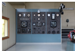
Hammeren hydro-electric plant Photo: Unn Yilmaz/NVE
